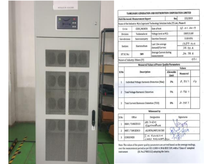
Power quality improvement
