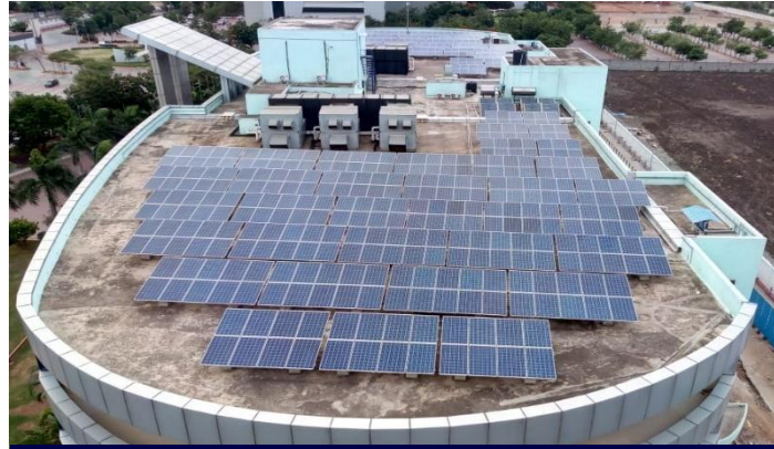
Roof top solar (750 kWp)
