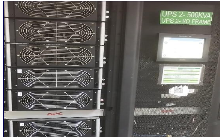
100% - Modular UPS (Efficiency - 99%)
