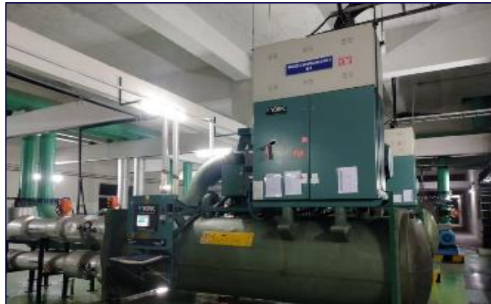
100% - Water cooled chillers ( kW – 0.65 kW/TR)
